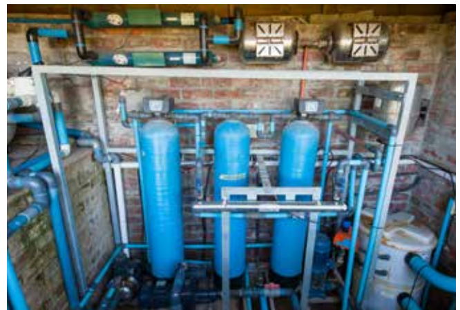
Pump room and water filters
